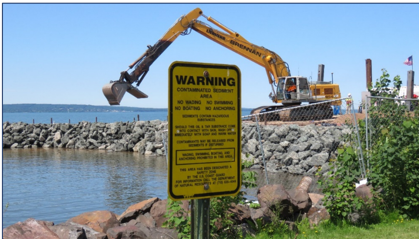
Figure 1. Operations begin along Lake Superior’s Chequamegon Bay, restoring a site known for contamination back to quiescence.
