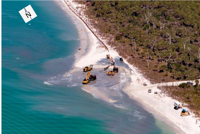
Figure 17. Aerial of CSSZ placement on 21 February 2015, approximately at Mid-placement construction, courtesy of GLDD (Brutsche et al, 2019).
