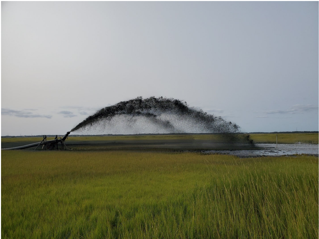
Thin-layer placement for habitat enhancement on Gull Island, NJ during navigation dredging.
