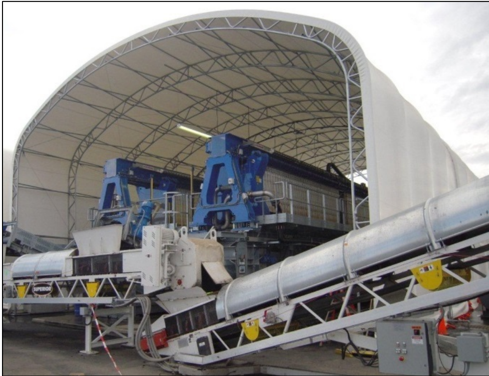
Figure 13. MFPs installed at UPF
