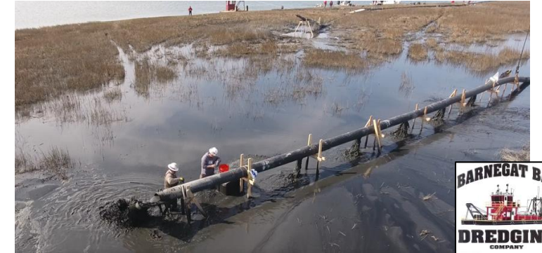
Sediment Distribution Pipe, Seven Mile Island Innovation Laboratory; with Barnegat Bay Dredging Company
