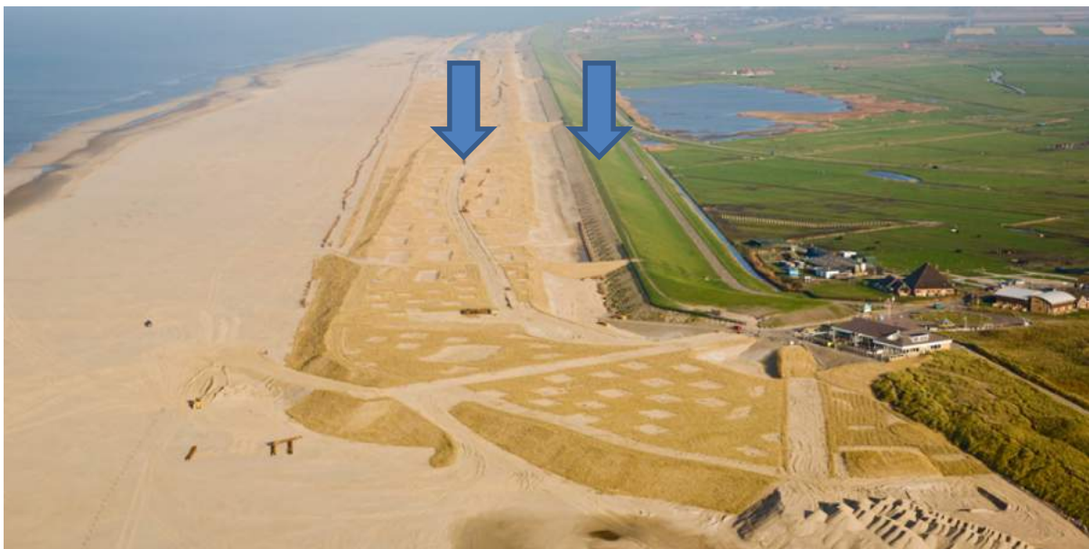
Innovative step change: from hard dike protection (right arrow) to a sandy solution (left arrow)
