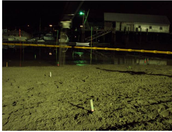
Figure 13. Precision placement of the sand cap with grade control survey stakes showing remaining 6 feet of surface gravel needed.
