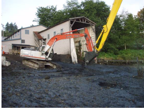
Figure 8. Transferring dredged sediments from the long reach to the excavator to the staging area.
