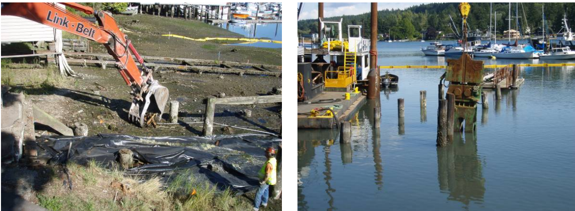
Figure 4. Extraction of timber piles using land-based excavator (left) and vibratory hammer (right).
