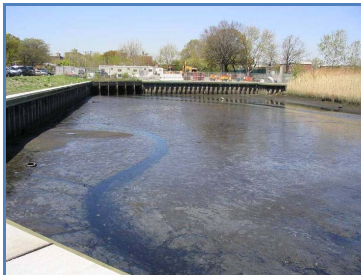
Figure 7. Mean low water condition exposes collected CSO sediments within Hendrix Street Canal.
