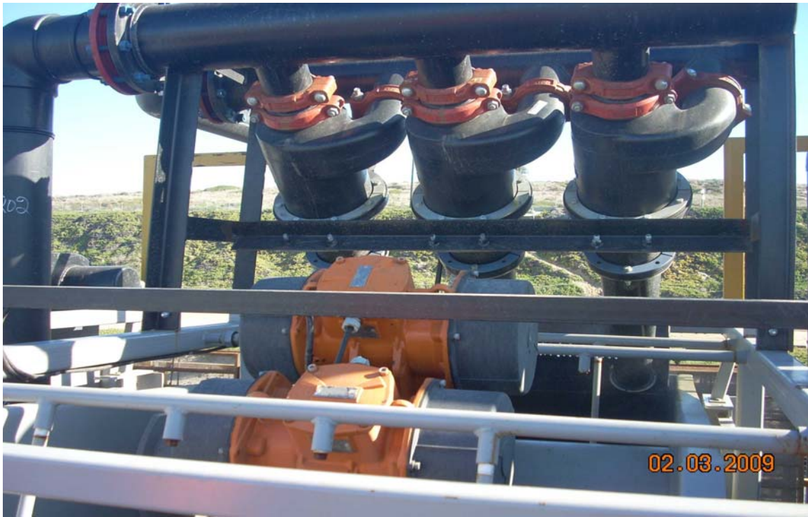
Figure 4. Hydrocyclones Mounted Above Linear Vibrating Screens
