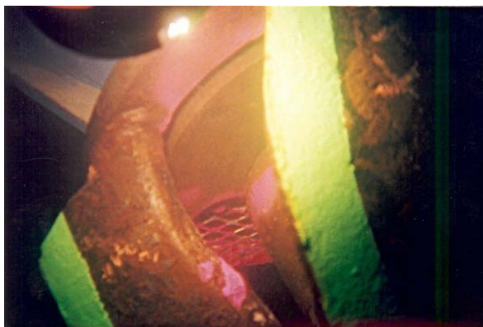
Figure 14. View of screened suction entrance between cutter blades.
