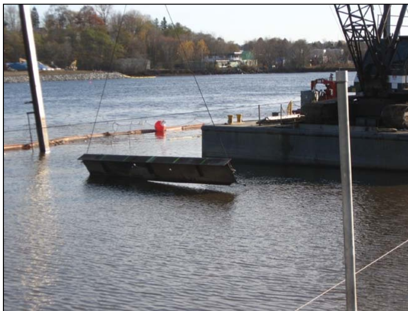
Figure 3. Using a steel beam drag bar to grade the surface of the cap.
