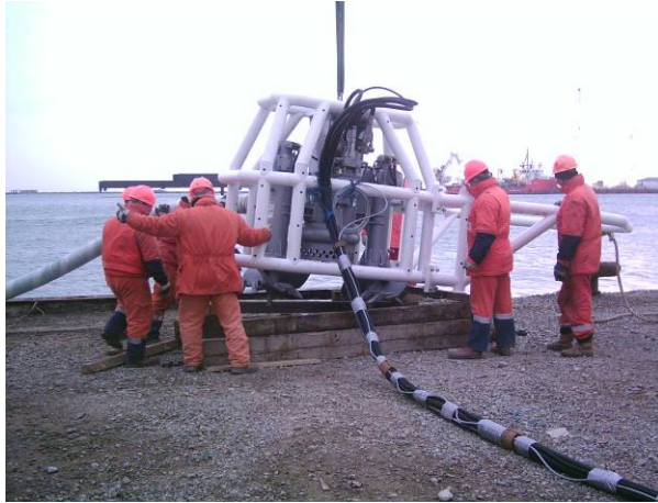
Figure 20. Off-Shore protective frame
