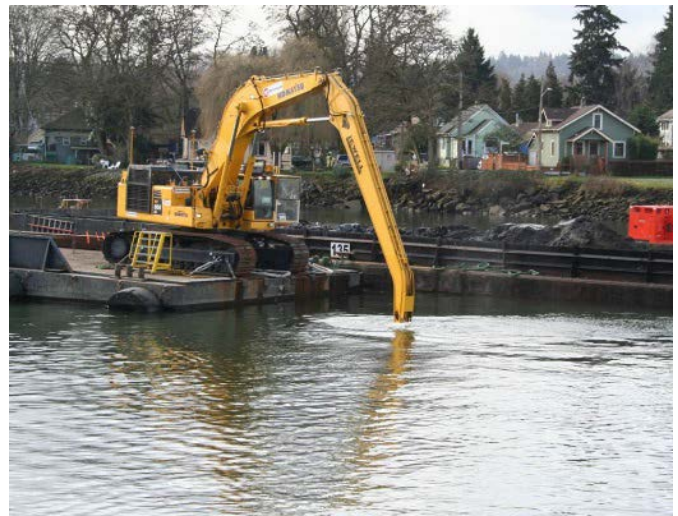
Photo 16 – Working in the “backyard” of local residents 24 hours per day required committed coordination.
