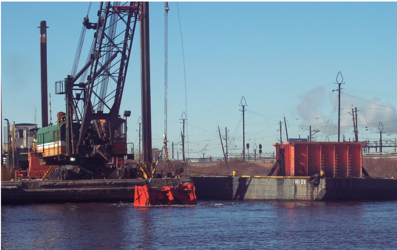
Bucket dredge using a Cable Arm ® clamshell in the Lower Passaic River, NJ.
