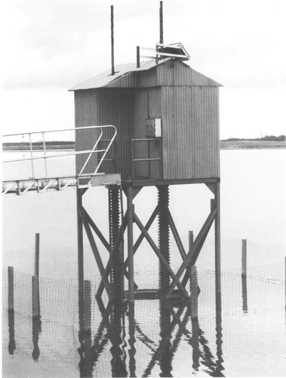
Figure 3. Photograph showing the telescoping weir, walkway, and wire mesh fence for floating debris
