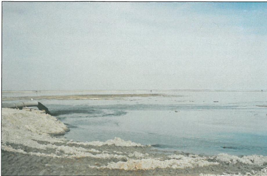
Discharge from a Hydraulic Pipeline
